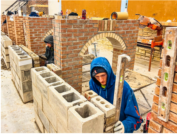
3rd Year PCC Apprentices Alex and Zachary Johnson building a brick and block project featuring a soldier detail.
